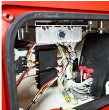
Electric cabinet is easily accessible.
